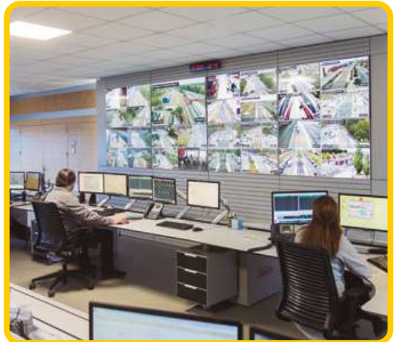
CCC – Central Control Centre
